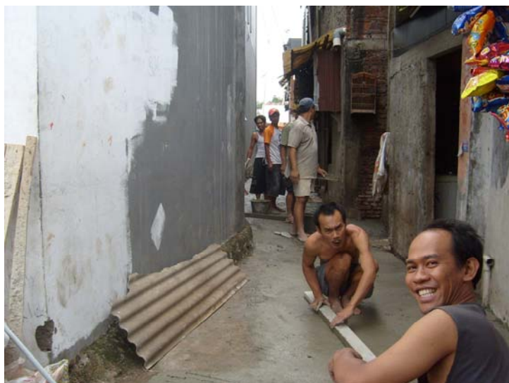
Paving an alley in an older section of South Jakarta – even the poorer parts of town are looking better.
